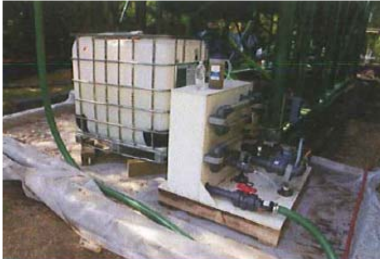
Figure 13. Portable polymer injection system.
