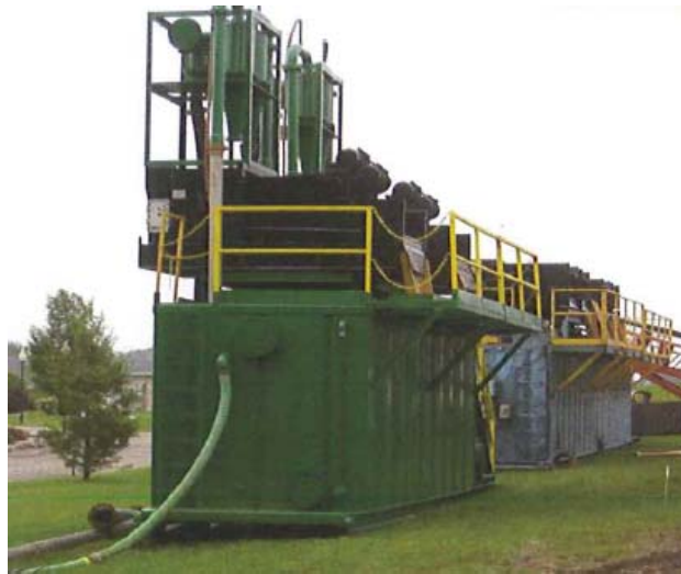
Figure 5. Placement of two additional components for screening and hydro cyclones.
