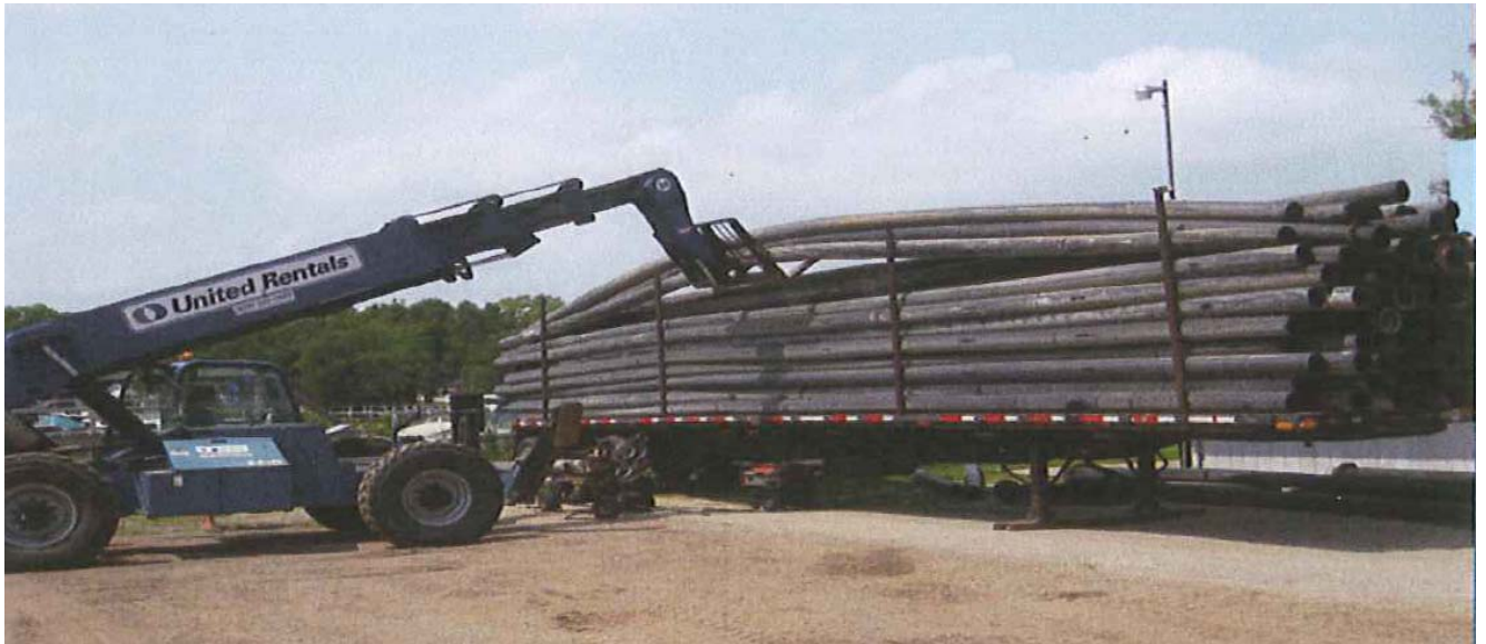
Figure 4. Unloading of HDPE dredging pipe used for pumping sediment and return water to the lake.
