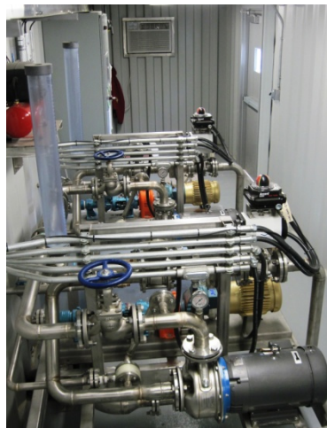
Figure 3. Emulsion polymer makedown system.
