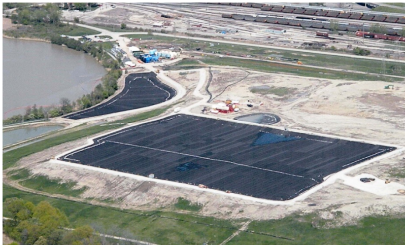
Figure 1. Aerial view of the site during construction of the sediment dewatering pads; the larger non-TSCA pad is in the foreground.
