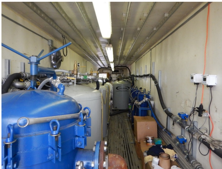
Figure 12. Water treatment plant within the SPA.
