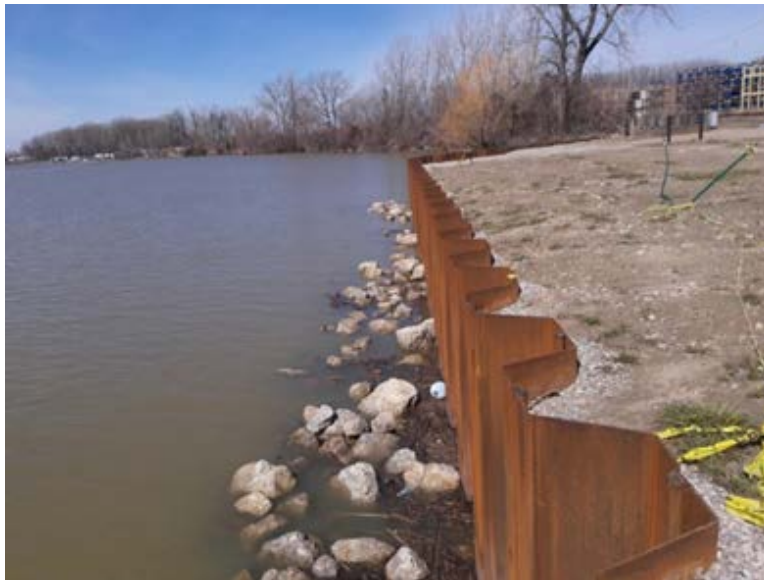
Figure 3. Installed sheetpile wall adjacent to NAPL Area (prior to dredging in the NAPL Area).
