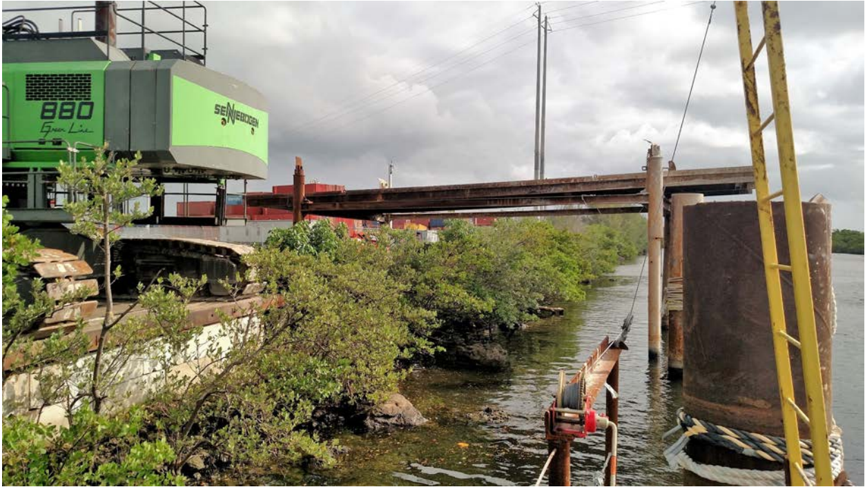
Figure 3. Shoreline Steel Spill Plate at the DMMA Offloading Area
