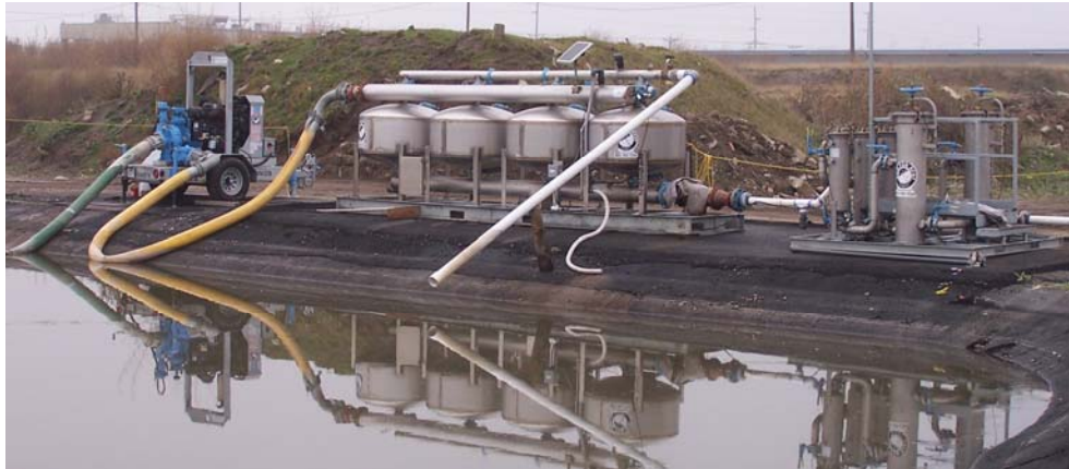
Figure 5. Sand filters (center) and bag filters (right) prior to discharge to waterway.
