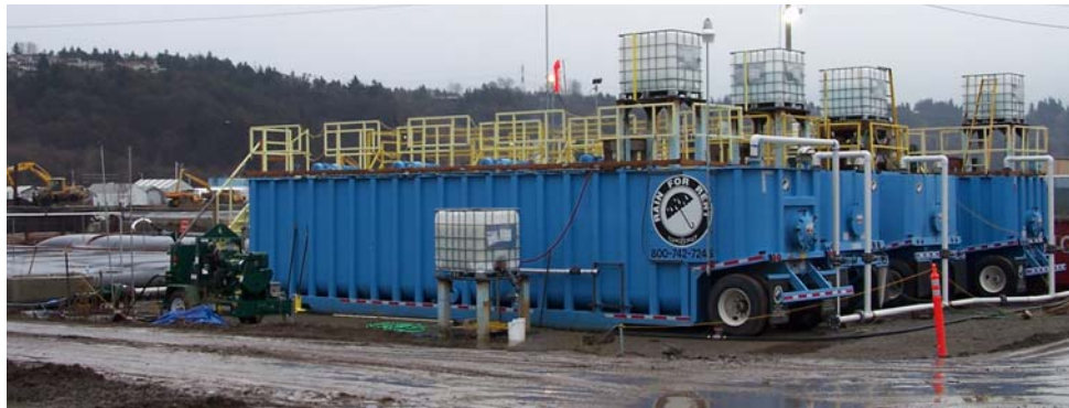
Figure 3. Mixing tanks, upland sediment capture system.
