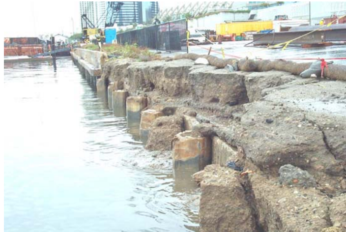
Figure 10. Typical portion of existing seawall in need of repair.
