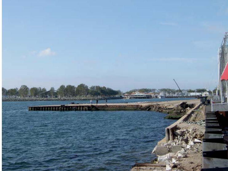
Figure 3. Campbell Shipyard project site before construction – seawall (right foreground) and south mole pier (center).
