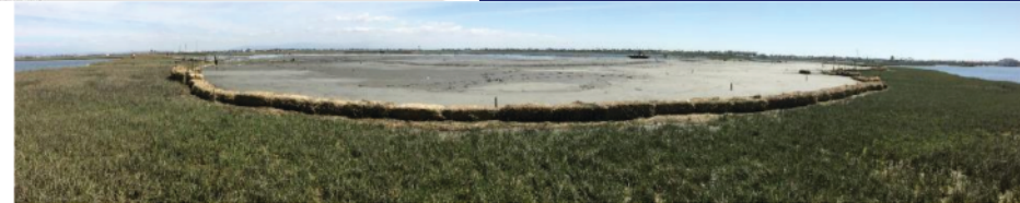
A thin layer (8-10 inches) of clean dredged sediments was added to 8 acres of a low elevation salt marsh within the Seal Beach National Wildlife Refuge in Orange County, CA.
