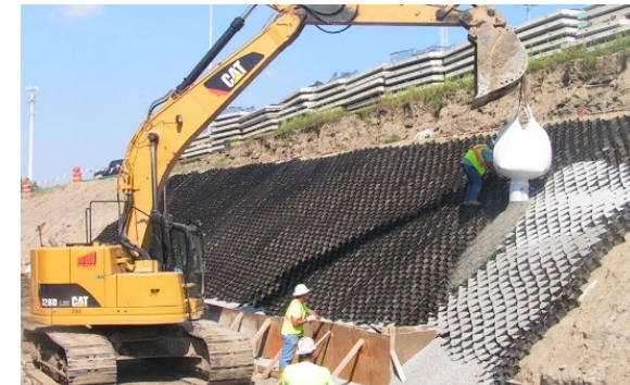
Seal Slope Seepage
