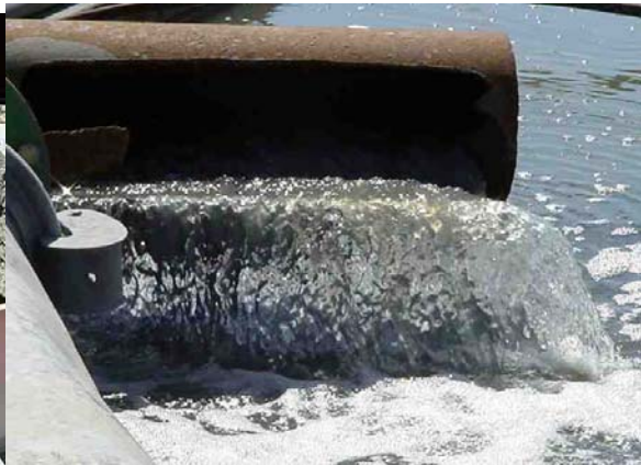
Figure 13. Effluent discharge returning back to the marina
