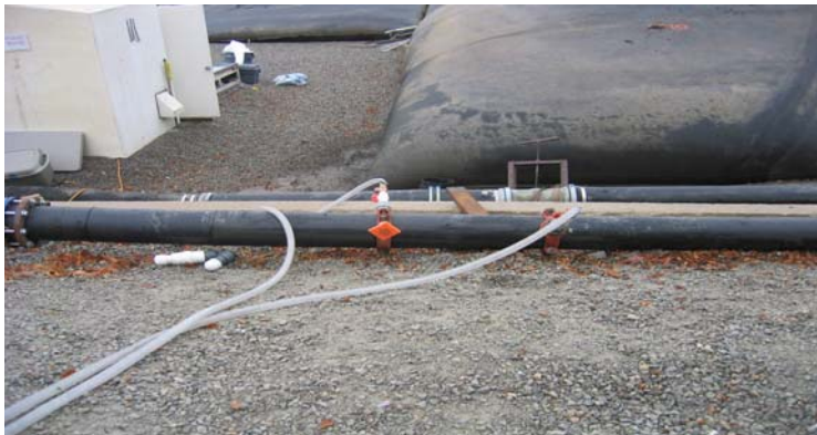
Figure 18. Polymer addition point into 2 slurry pipelines
