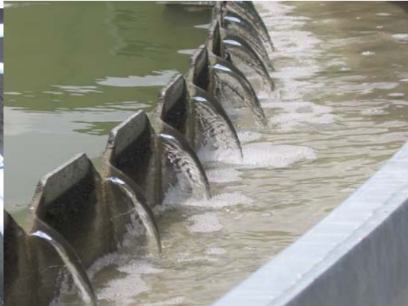
Figure 23. Gravity thickener overflow weir
