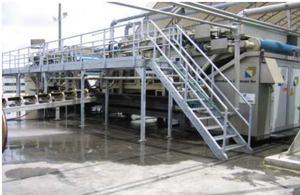
Figure 24. Belt filter presses for dewatering thickened solids from thickener underflow
