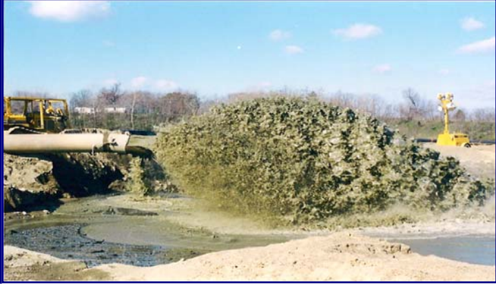
Figure 7. Slurry pipeline discharge into primary containment area
