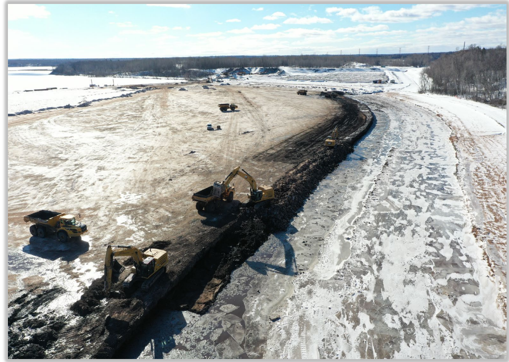
Mechanical dredging above OHWL portion of the area to become a new shallow sheltered bay
