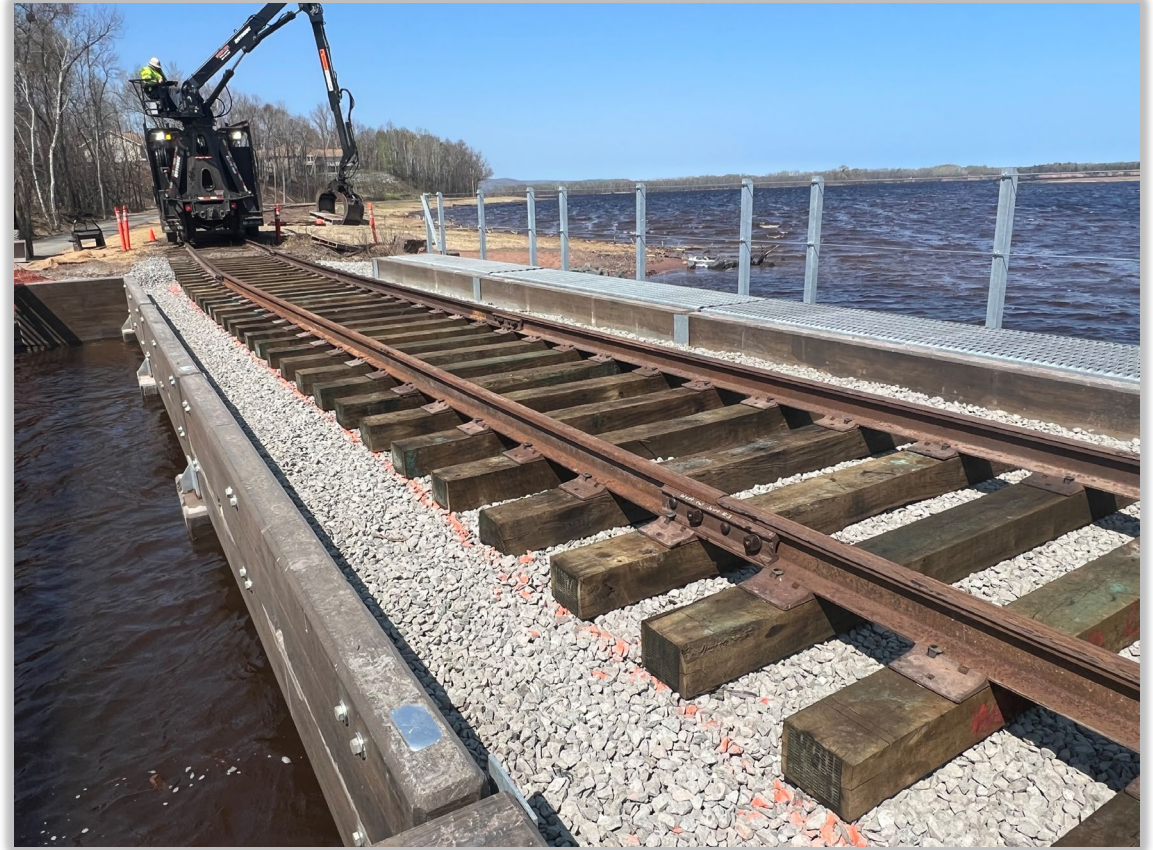
Construction of the new railroad bridge at the opening of Unnamed Creek and the new shallow sheltered bay
