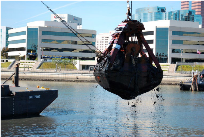
MCC's Derrick Valhalla dredging in Long Beach, CA with a Round Nose Style Bucket
