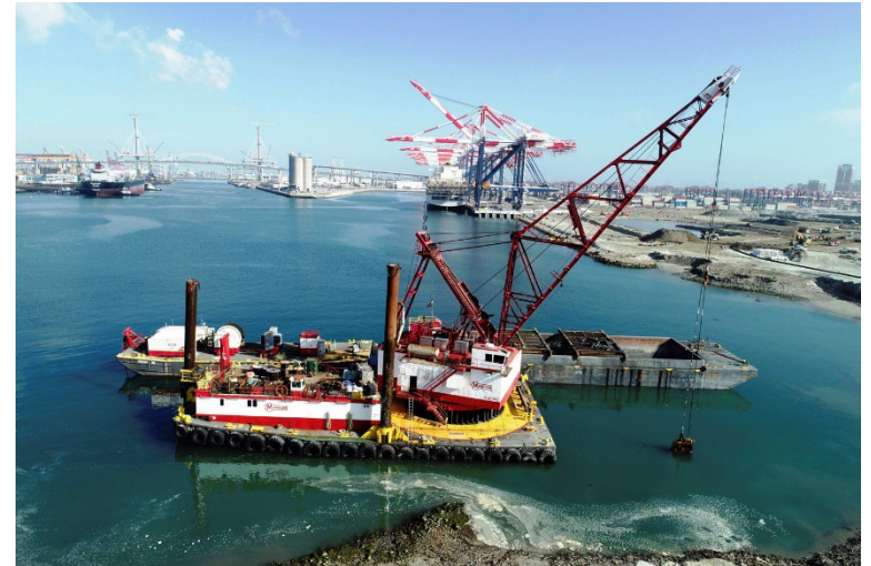
MCC's Derrick Njord dredging at Pier E Berth E22 Port of Long Beach, CA
