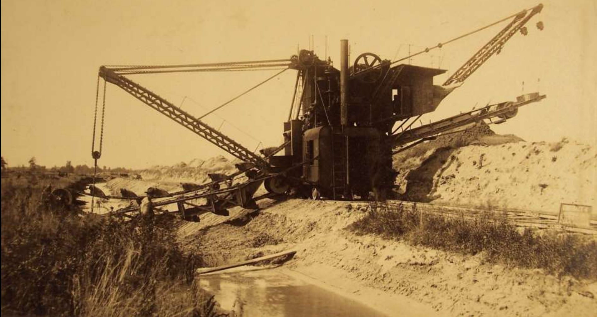
Neg. #5. Contract #4. Looking W. from Sta. 6800, showing work of Lubecker on prism excavation, Oct. 1, 1906.
