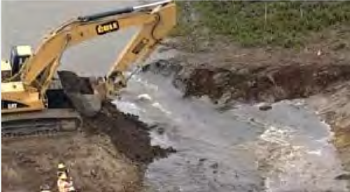
Levee Breached at Hamilton Airfield (KPIX)
