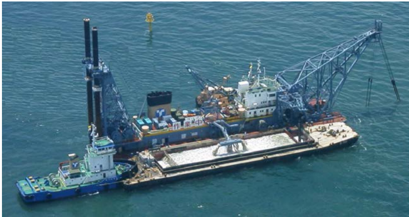
Barge loading system
