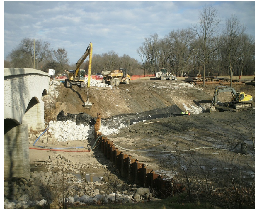
Restoration begins on the north bank on Zone 3A, trenching keyways, placing fabric and riprap (1/9/2012)
