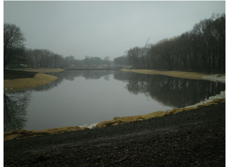
Water flow from Lincoln Creek was redirected through Zone 2A from Zone 2B
