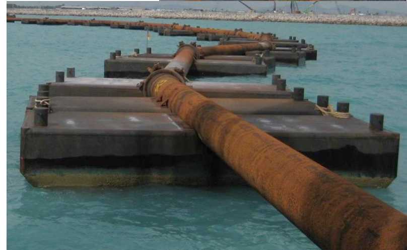
No flexibility in pipe connection
