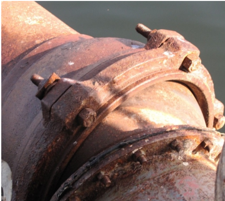
Rust on Ball Joint
