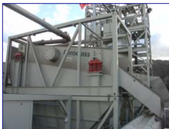
Figure 8. Sand separation module.
