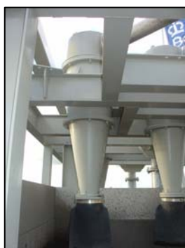
Figure 9. Hydrocyclones for sand separation.
