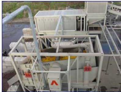
Figure 5. Screening stage equipment.
