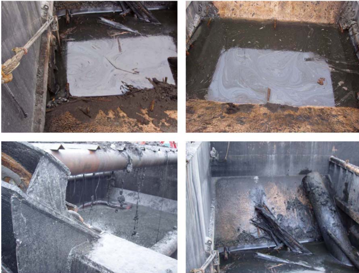
Figure 7: Photos documenting creosote-treated piling remnants and sheen accumulating in the disposal barge.
