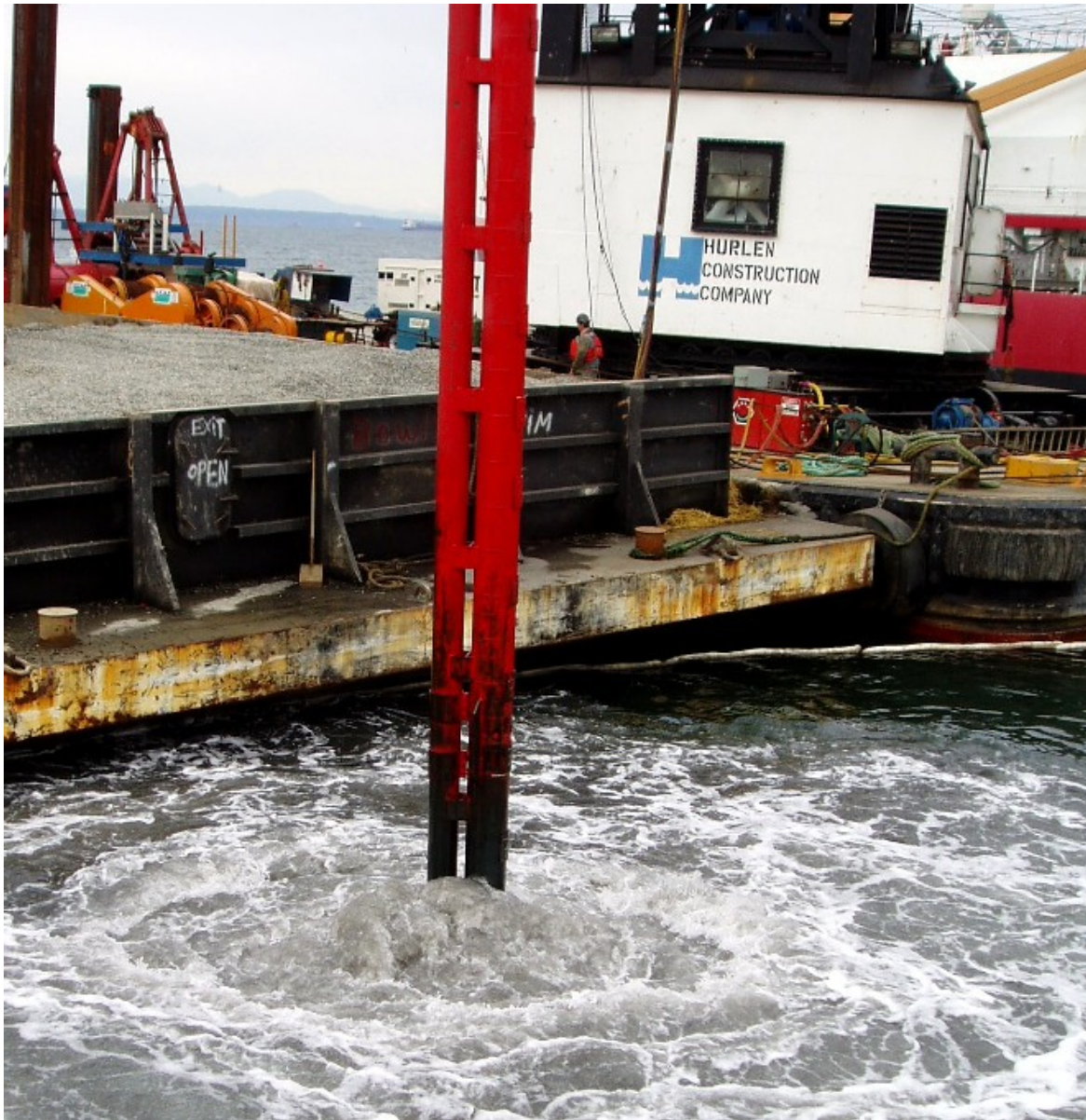
Figure 2: Gravel column construction is underway, as gravel is injected deep into the sediments. Note the water disturbance in the immediate vicinity of the probe.
