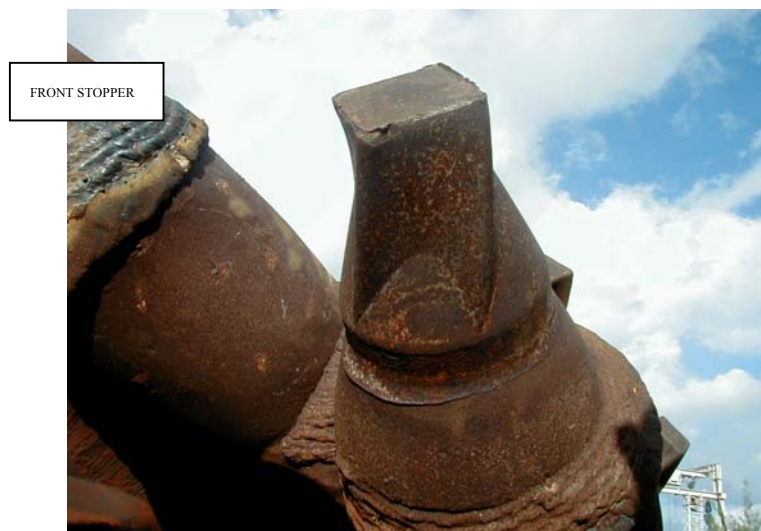
Figure 6. Wear on front stopper resulting in reduction of pretension on the locking
