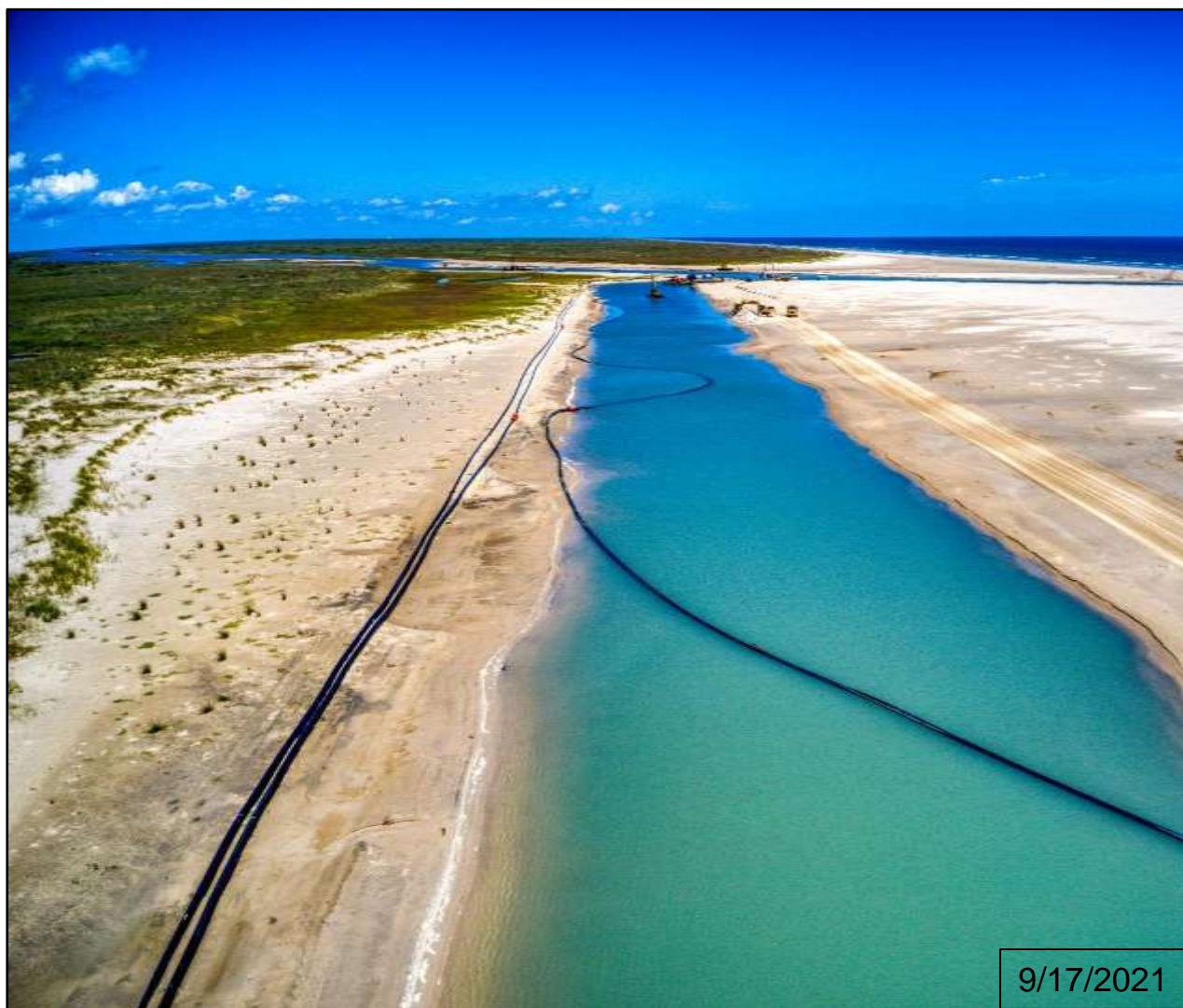
Pipeline transporting dredged material from cutter head dredges to disposal area.
