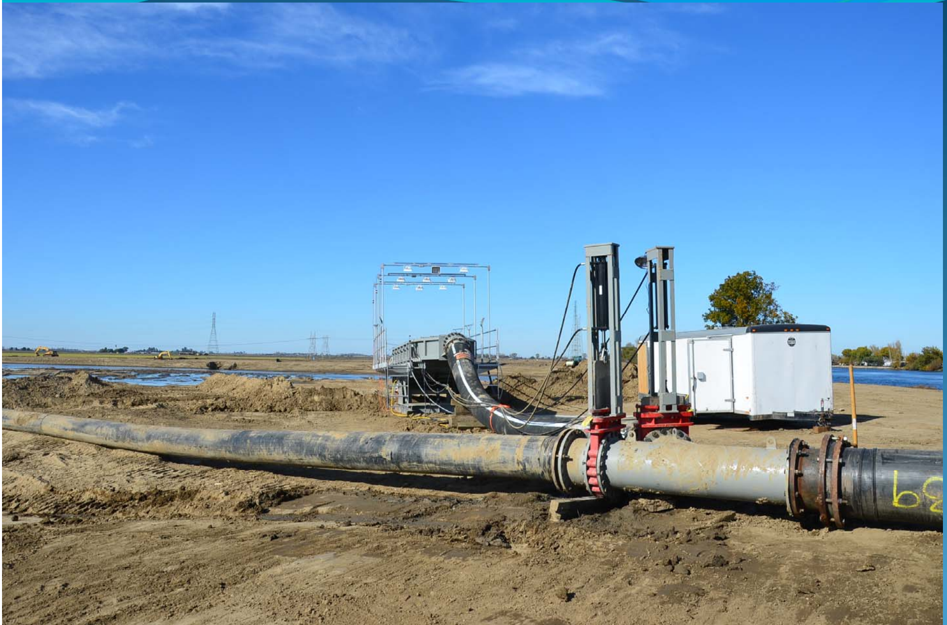
Port of Stockton Fish Entrainment Screen
