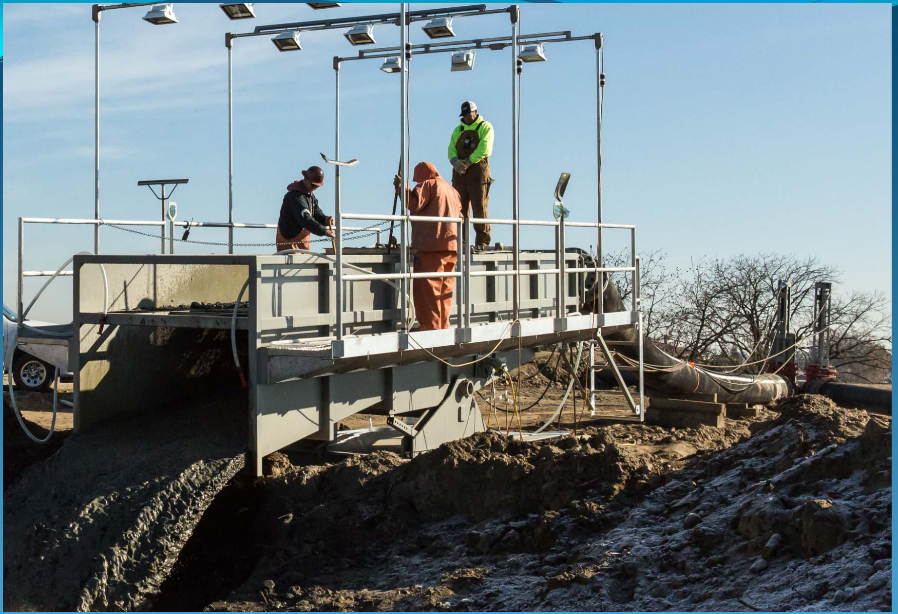
Port of Stockton Fish Entrainment Screen
