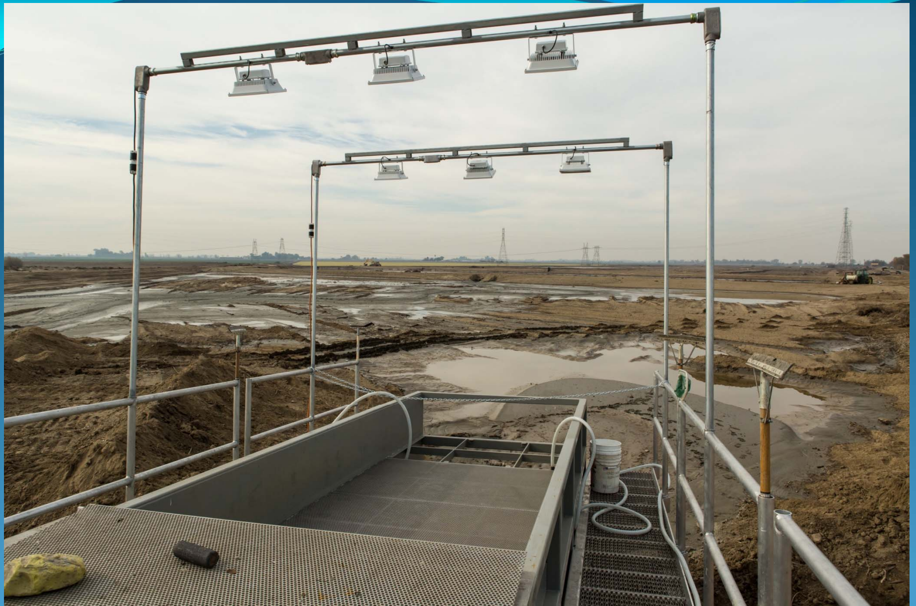
Port of Stockton Fish Entrainment Screen
