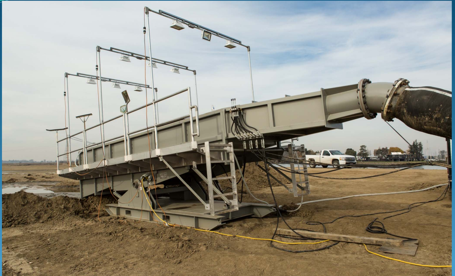
Port of Stockton Fish Entrainment Screen
